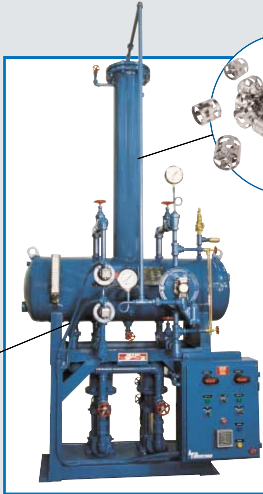
1,000#/hr. Deaerator system (2) B.F. Pumps Theatre installation
